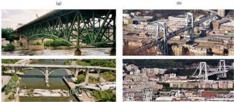
Fig. 1.1: Catastrophic failures of the I-35 W Mississippi river in 2007 (constructed between 1964 and 1967 in Minneapolis, Minnesota, US) (source: [7]) (a) and the Morandi Bridge in 2018 (constructed between 1963 and 1967 in Genoa, Italy) (source: EFE agency).
